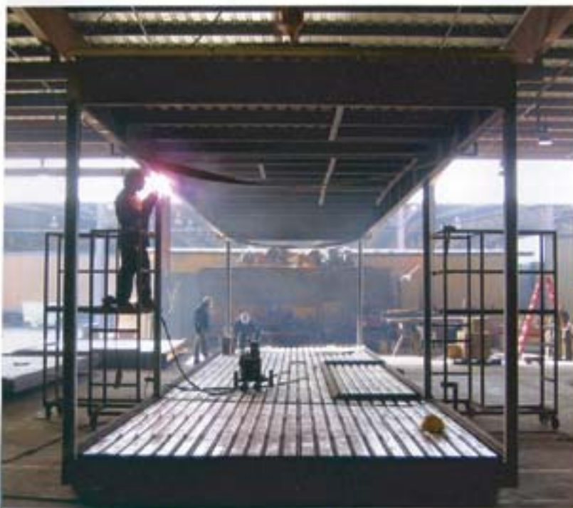
ASSEMBLY LINE. Inside Marmel Radziner's 65,000-square-foot factory, workers construct one of their models using a 12-foot module and eco-friendly materials. Top: Marmel Radziner's Desert House prototype in Desert Hot Springs is a prefab showpiece that has attracted much attention.
