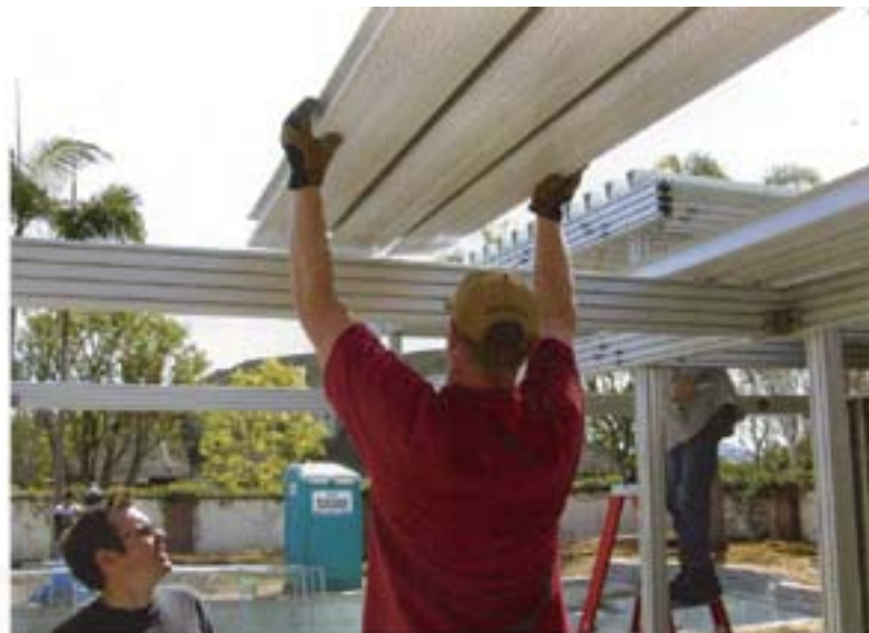
PANELIZED KIT. A construction crew assembles Taalman Koch's iT prototype, a striking, 1,100-square-foot aluminum-framed box with a steel roof that is almost entirely glass. Two others are nearing completion.
